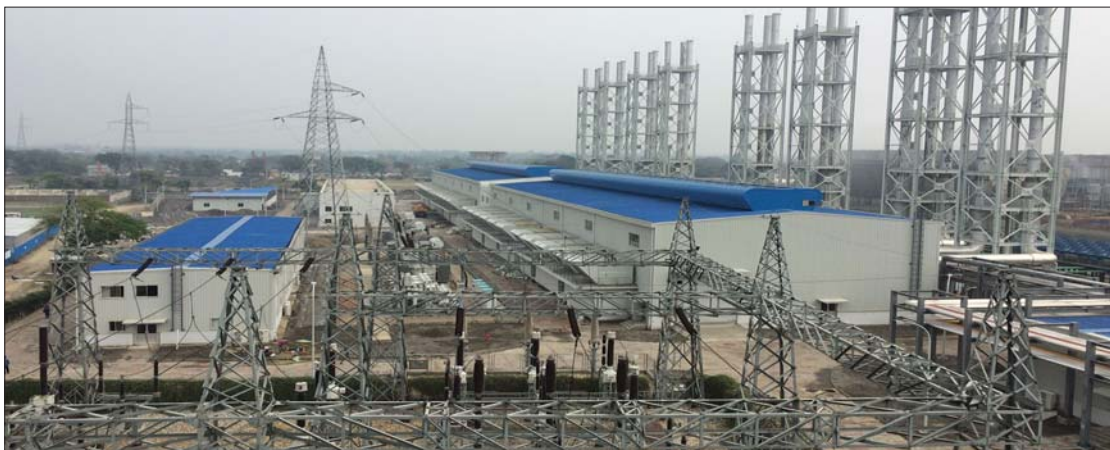
An OBL financed Power Plant
