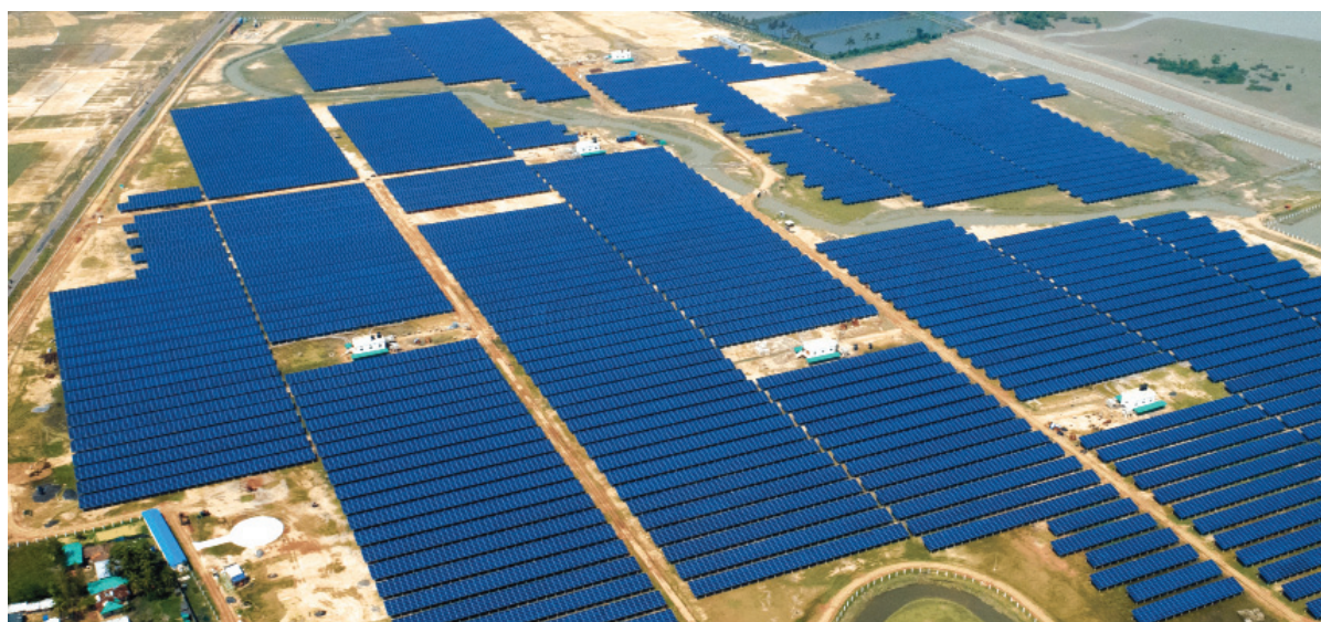
An OBPLC financed Grid Tied Solar Park
